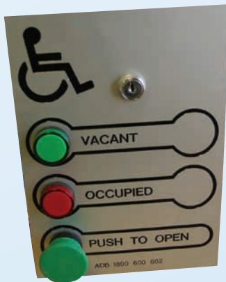
Push button control panel for entry with emergency key switch
